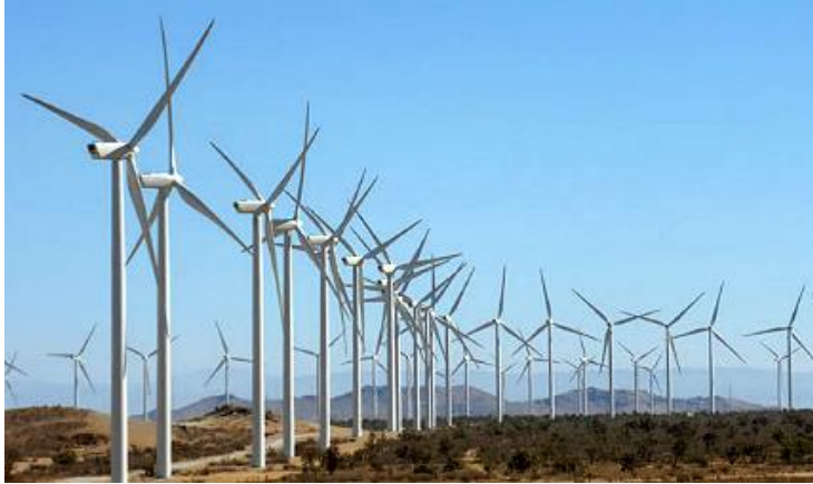
Figure 70. Alta wind Centre, Kern County, California U.S.A
