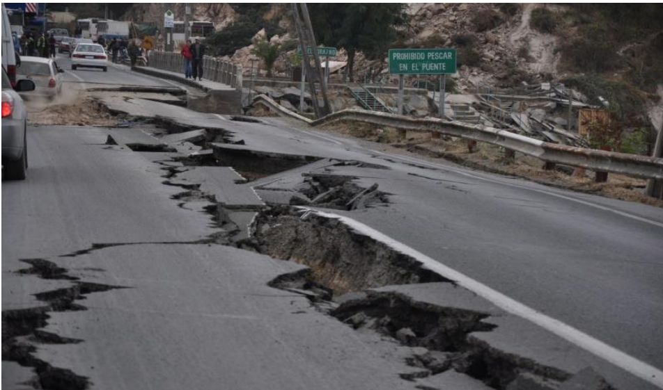
Figure 3.6 A road destroyed by an earthquake in Spain
